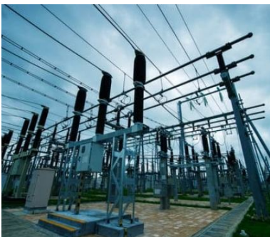
Substation Inlet and Outlet Lines
