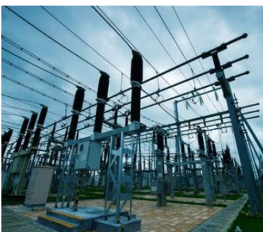
Substation Inlet and Outlet Lines
