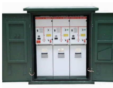
Cable Branch Boxes
