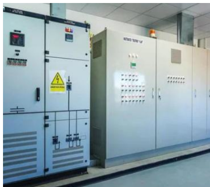
High and Low Voltage Switchgear
