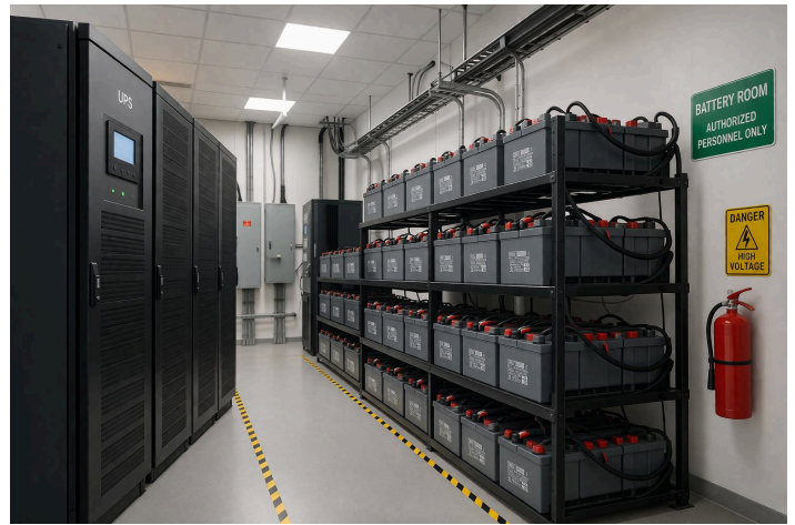
UPS Battery Rooms
