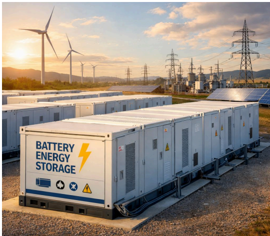
Battery Energy Storage
