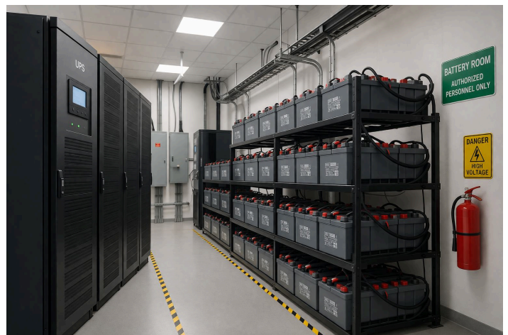
UPS Battery Rooms
