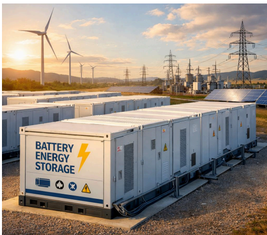
Battery Energy Storage
