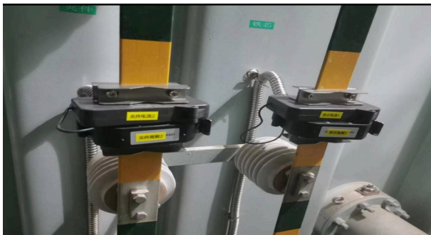
On-site installation diagram of high-frequency partial discharge sensor
