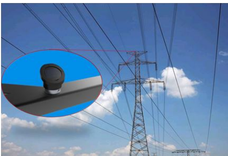
Transmission line tower
